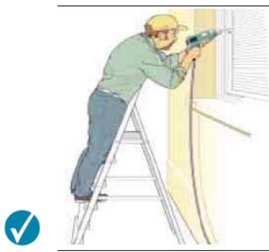
Correct – steps facing work activity
